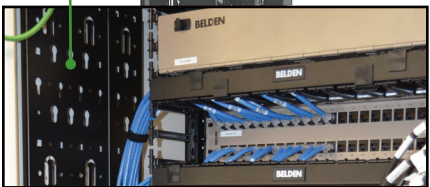
Lacing Panel shown in enclosure
