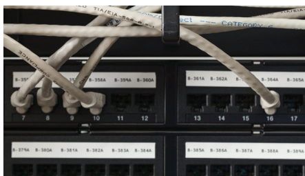
Patch Panel Labels
