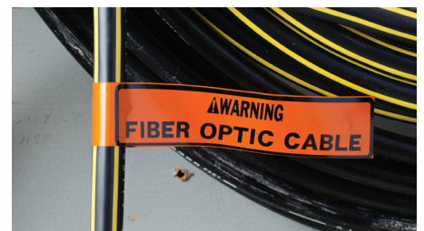
Fiber Optic Cable Markers
